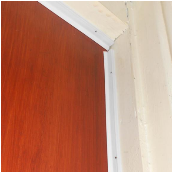
Draught proofing around door frame
