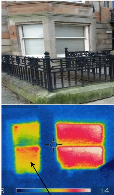
Less heat loss from this window with the thermal curtain
