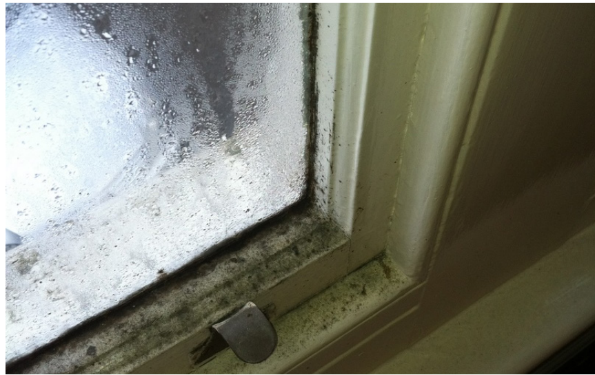
Mould caused by moisture build-up due to condensation
